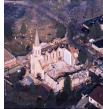
St. Anthony's under construction, with new construction inserted into the fragments or "ruins" of the old church.
