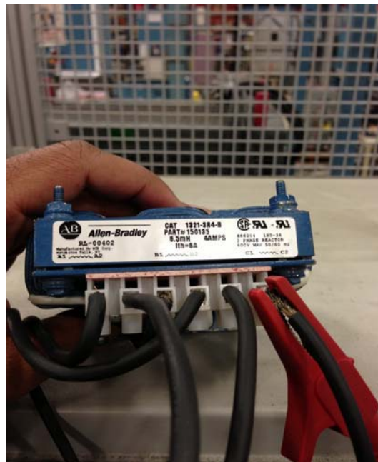
Figure 4.10: Line Reactor Used to Create Voltage Unbalance
