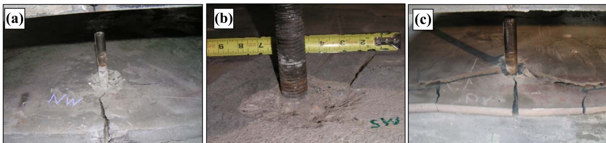
Figure 2.7 Post-test photographs showing (a) grout damage of 19 mm [0.75 in.] diameter anchor Test; (b) concrete damage of 31.8 mm [1.25 in.] diameter anchor and (c) grout damage of 31.8 mm [1.25 in.] diameter anchor
