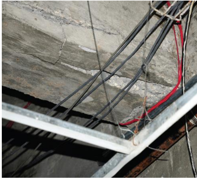
Fig. 2.5 Damage to the beam near the beam-wall connection in Haiti Earthquake in 2010
