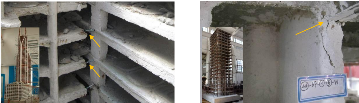
a) failure of connections between adjacent buildings. b) failure of girder-wall connection.
