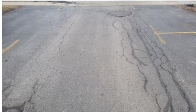
Figure 2.12: Rutting Damage Caused by Traffic Loads
