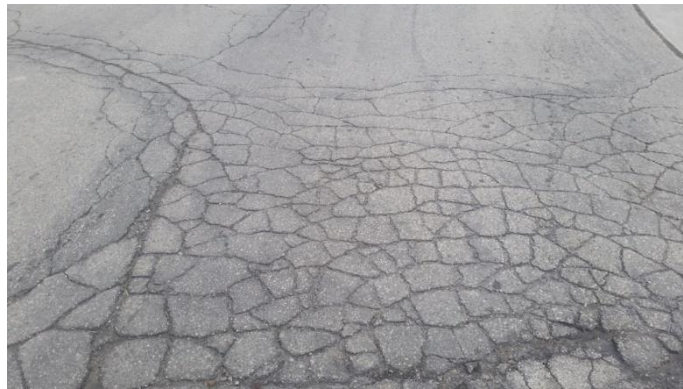
Figure 2.13: Asphalt Fatigue (Alligator) Cracking
