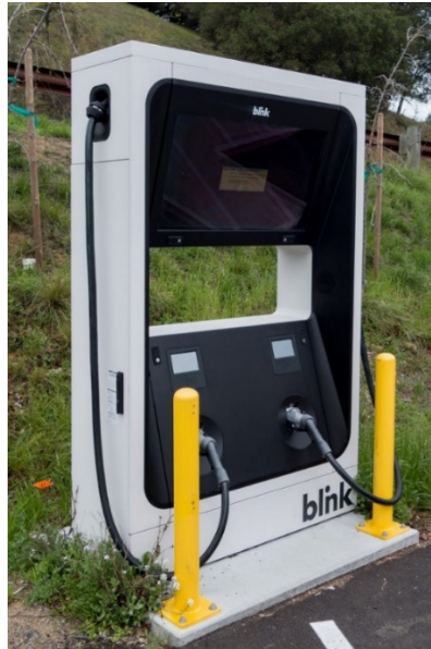
Figure 1-5. A picture of a DC fast charger.
