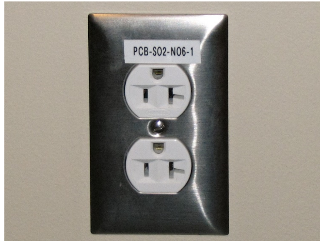
Figure 1-2. Standard Household Outlet-Charging
