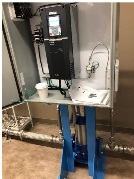
Figure 14- Pump's safe mode controller
