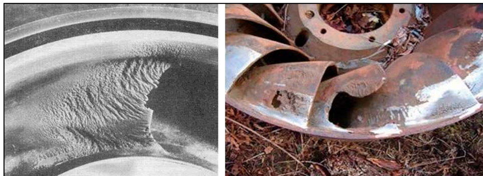
Figure 5: Severe cavitation erosion as witnessed on a Francis turbine [10]
