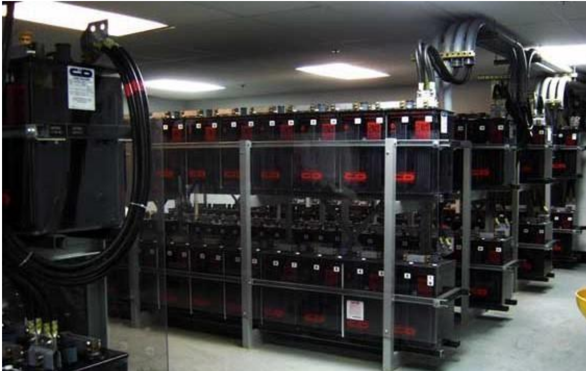
Fig. 1.7 – Representative Image of Stationary Batteries [11]
