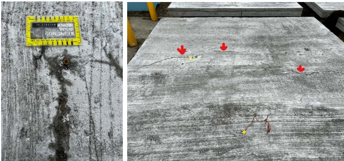
Figure 20 Cracks on Overlay Slab 7 (NC-I)
