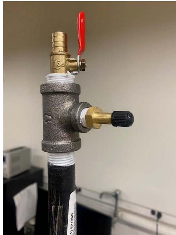
Figure 3.6: Schrader and ball valves connected to the top of the tank structure.
